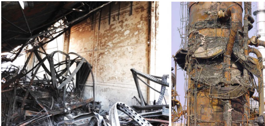
Fig. 8.1 Example of creep in metallic structures affected by fire. Notice that most of the structural components deformed and collapsed under their own weight
